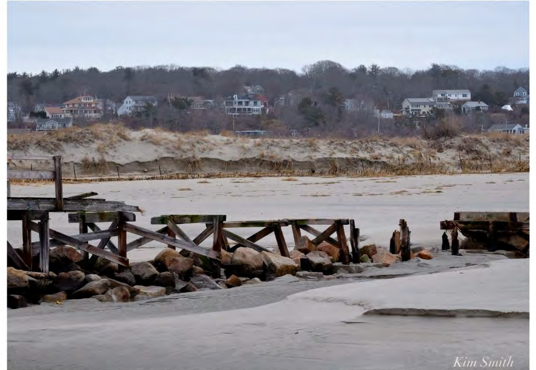
Kim Smith. Good Harbor Beach Footbridge damaged . 2018. Good Morning Gloucester .
